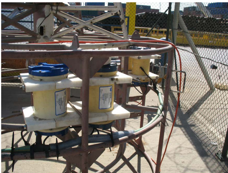
Figure 6. Cables Protected with Hose
