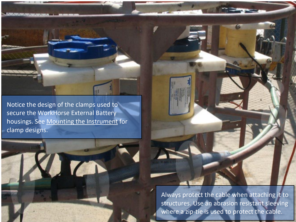
Figure 12. Cables Protected with Abrasion Resistant Sleeving
